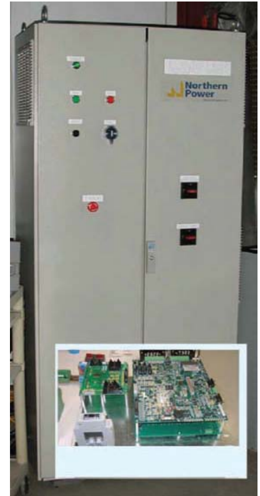
Interconnection switch and control board (Source: Kroposki, et al. 2008)
