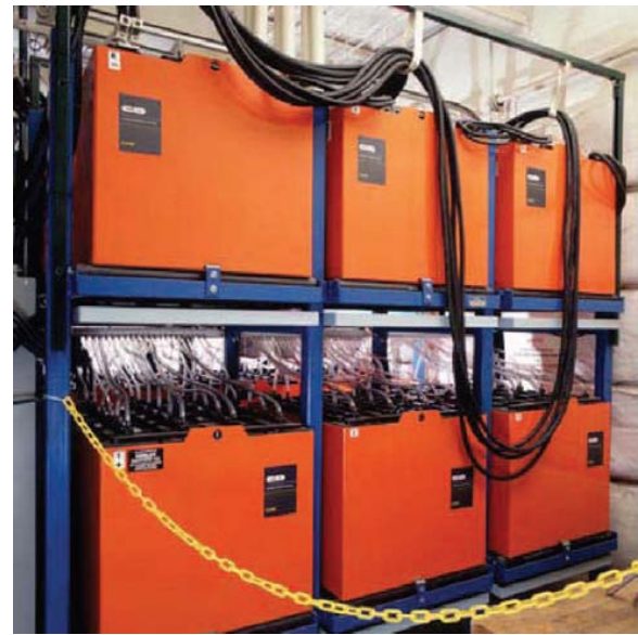
Large lead-acid battery bank (Source: Kroposki, et al. 2008)
